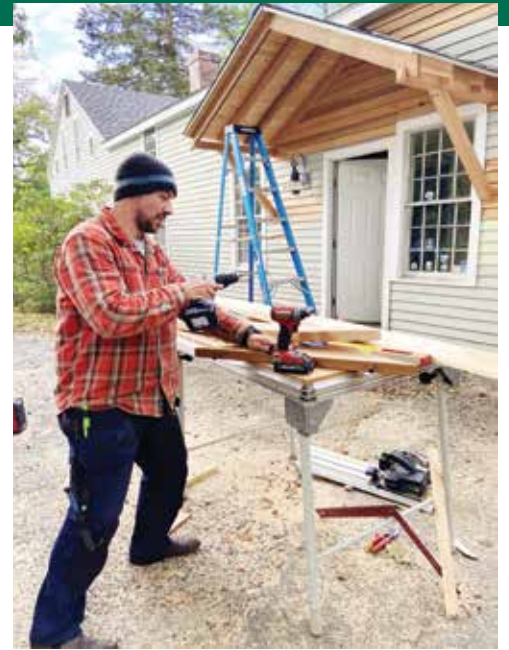
Local craftsmen have now completed the new entryway at Mount Grace's headquarters, Skyfields Arboretum.
